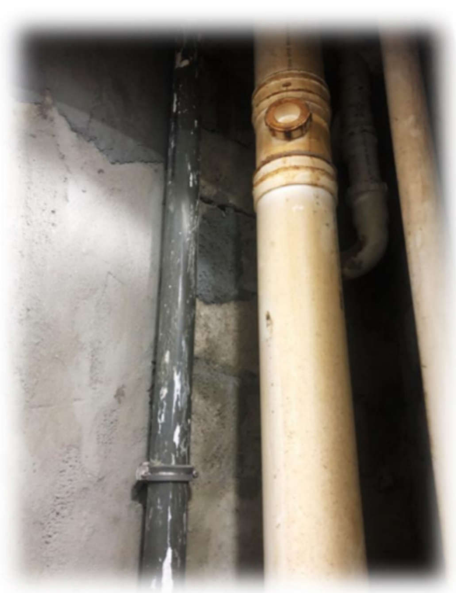
Internal pipe duct accessible from common parts
